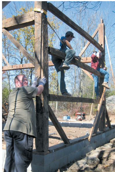
Friends and neighbors of the Shipman family on the corner of Baseline and Fix roads built fellowship as they built an 1800s carriage house.
